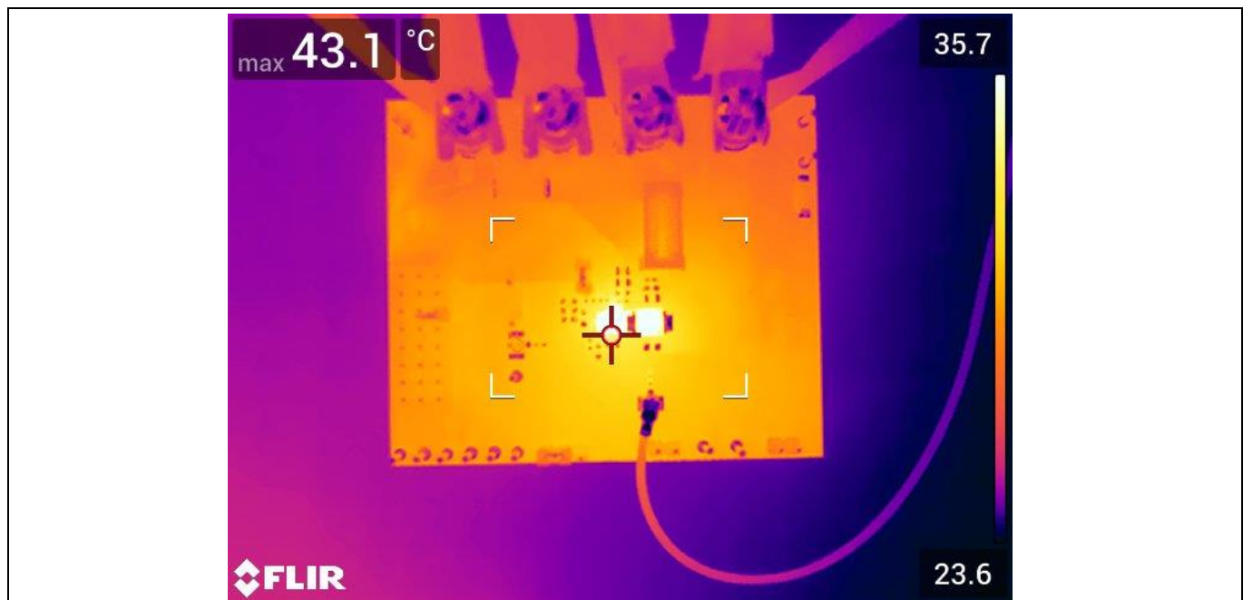
Figure 17 Thermal image of the board at 3 A load IR3823A = 43.1°C, F_{sw} = 1000 kHz, T_a = room temperature, natural convection
