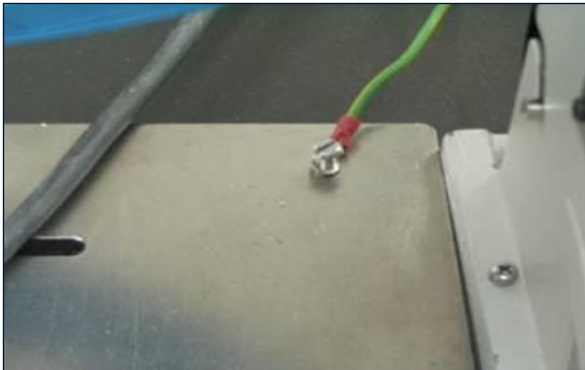
Grounding Wire Not Secured
