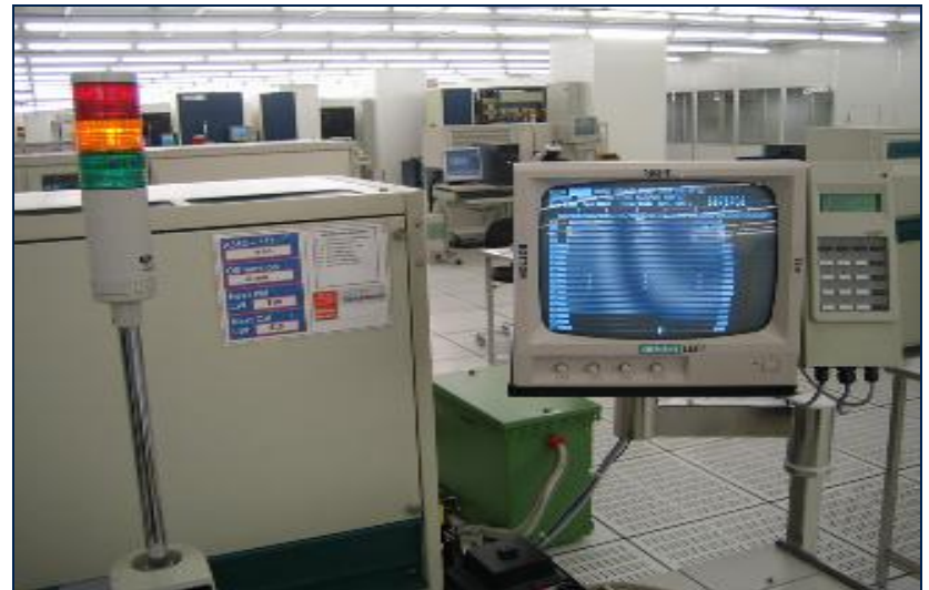
Tower Light Faulty
